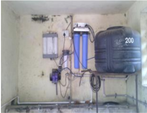
RO Plant used at Andhatri PS
