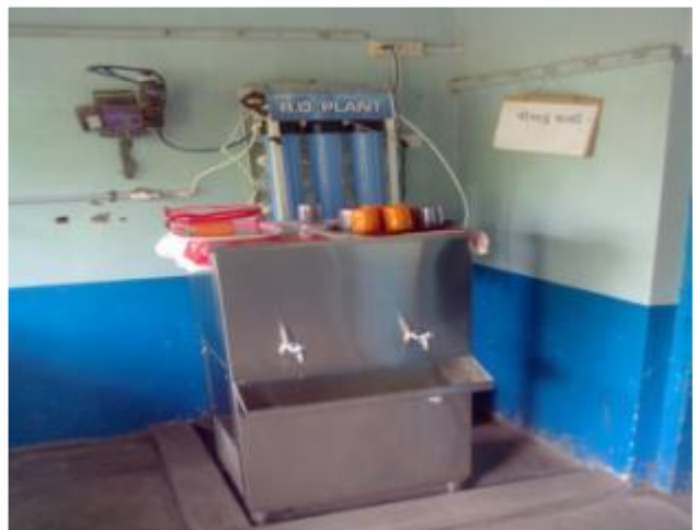
RO plant with water cooler at Choryasi Lavasa PS
