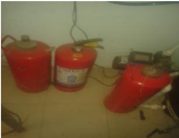
Fire extinguishers at Movasa PS
