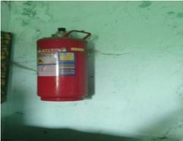
Fire extinguishers placed at Pinchipur PS
