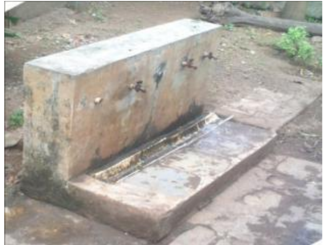
Poorly managed water facility at Moskut PS
