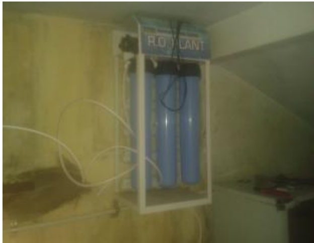
RO machine used for drinking water at Simalgam PS
